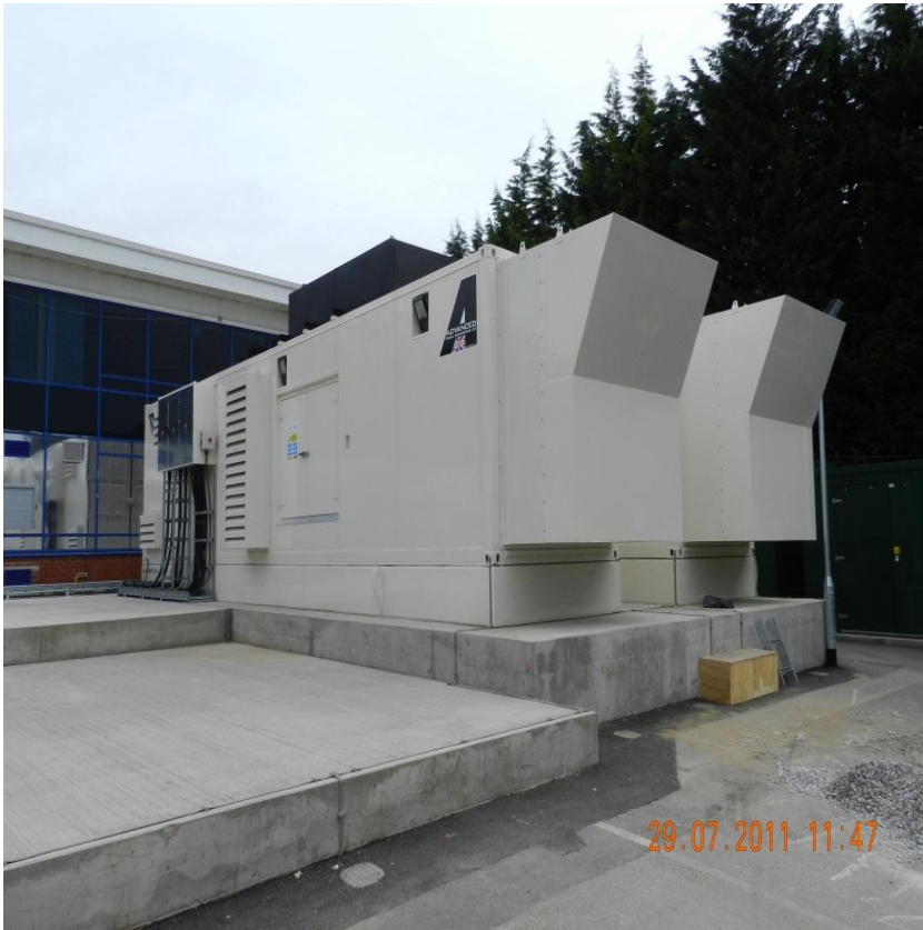
Co-op Bank Data Centre 2 x 500 kVA
