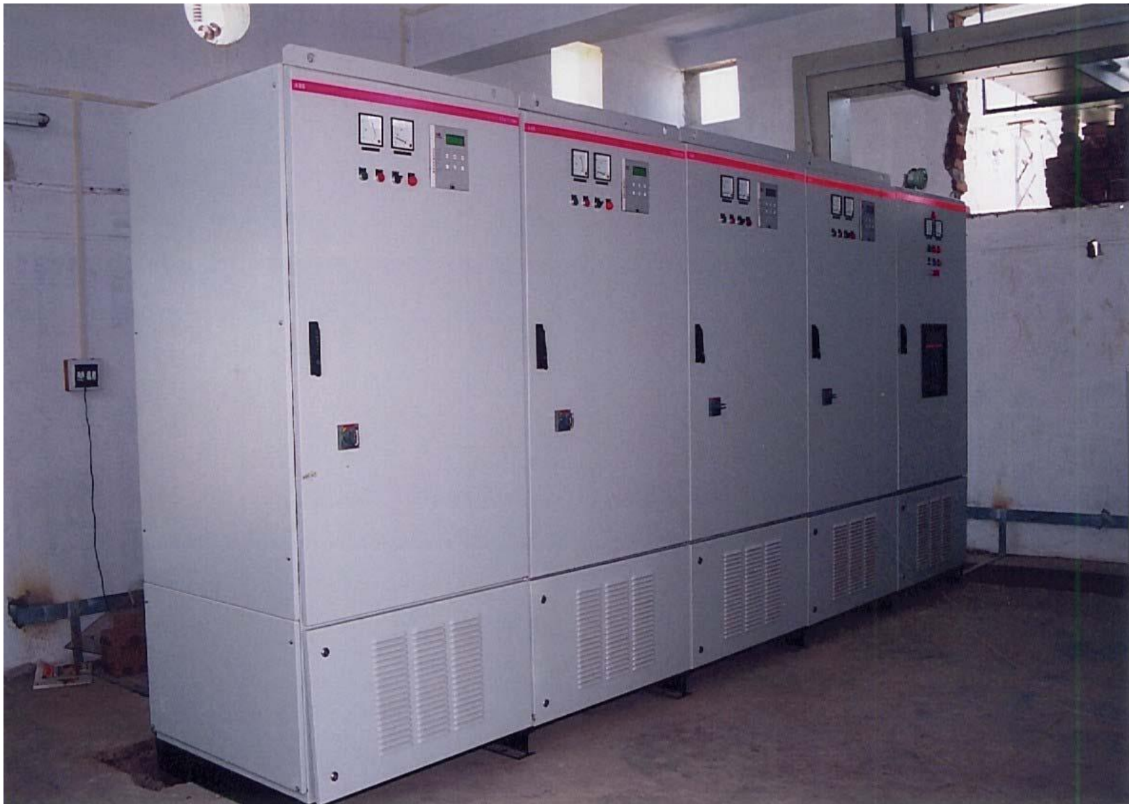
ABB's 3 MVAR DRPC system at Lasalgaon CR substation (1800 kVAR detuned HT FC + 150 KVAR*8 LV side 430 V Statcon)
