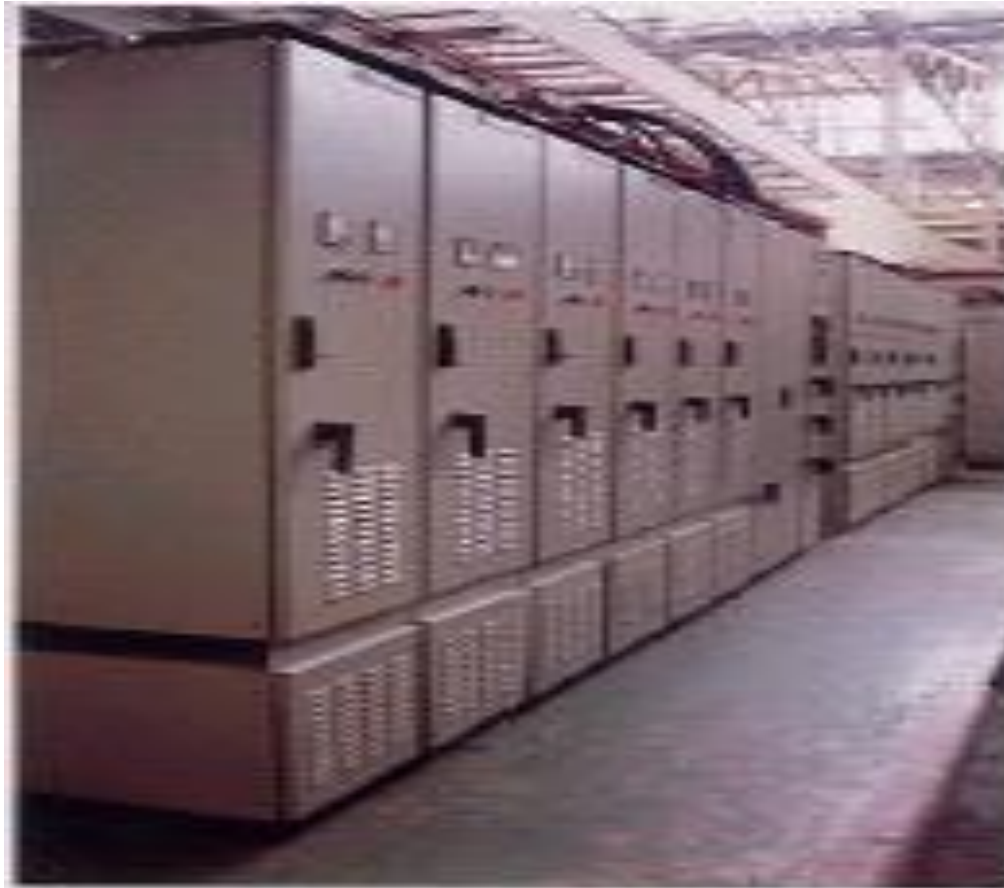
ABB's STATCON installation ( 3 \times 600 \text{ kVAR} = 1800 \text{ kVAR} ) at TELCO, Pune, for spot welding application
