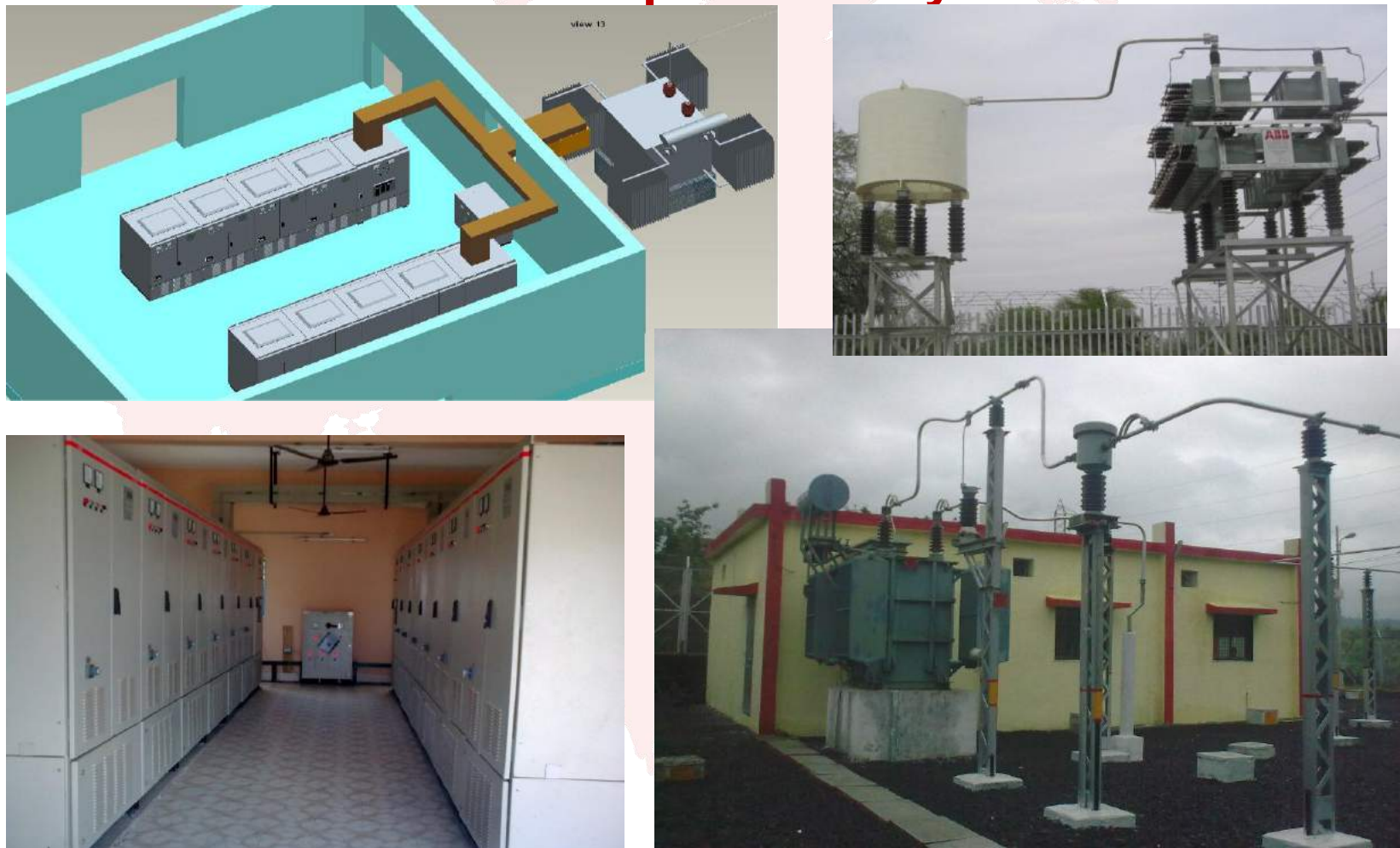
Figure 20 : Typical Railway STATCON + MV Capacitor Bank Installation
